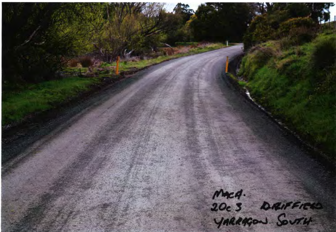
Construction with 20 mm VicRoads Class 3 crushed rock. Photo provided by Ross Kennedy
