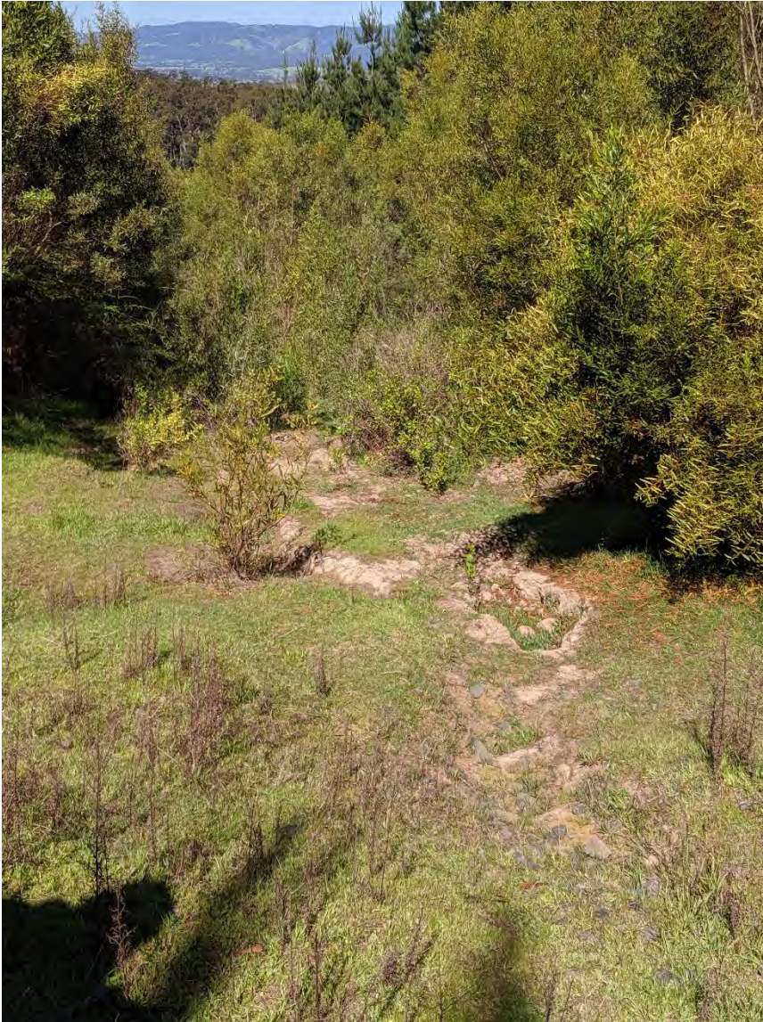
View to east from WTG38 location showing irregular ground surface with some evidence of shallow erosion
