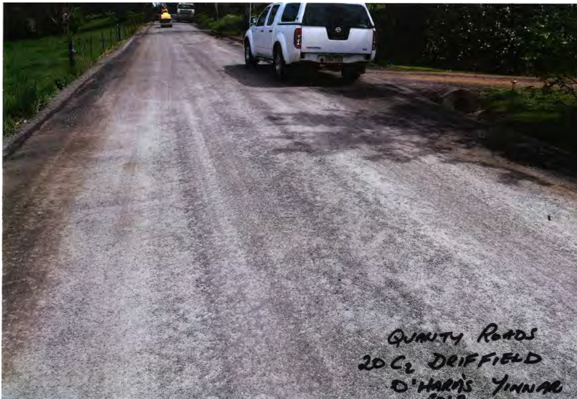
Road construction using 20 mm VicRoads Class 2 crushed rock. Photo provided by Ross Kennedy.
