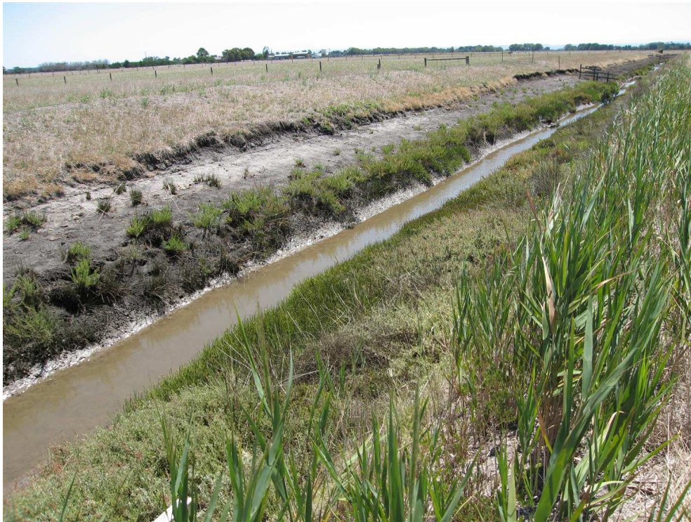
Plate 7. Healesville – Koo Wee Rup Road Upgrade: view from east to west bank of McGregors Drain and upstream of South Gippsland Highway, looking north (February 2008).
