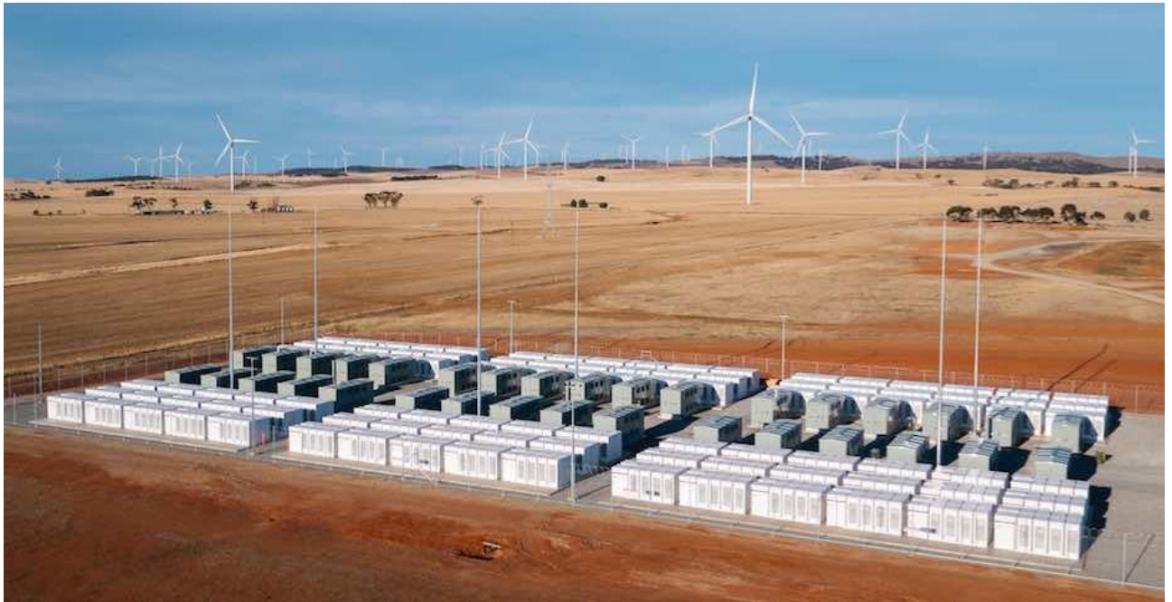
Figure 3-6: Typical battery storage
