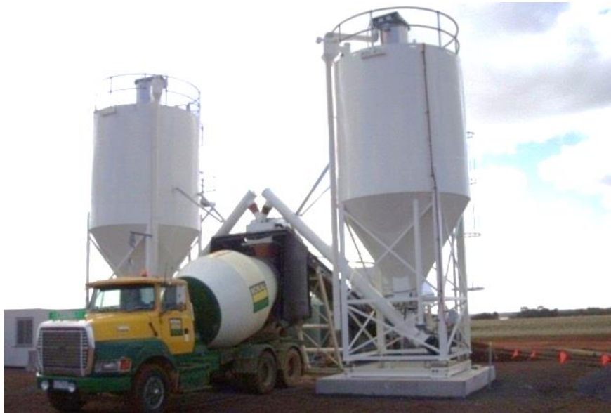
Figure 3-8 Portable batching plant
