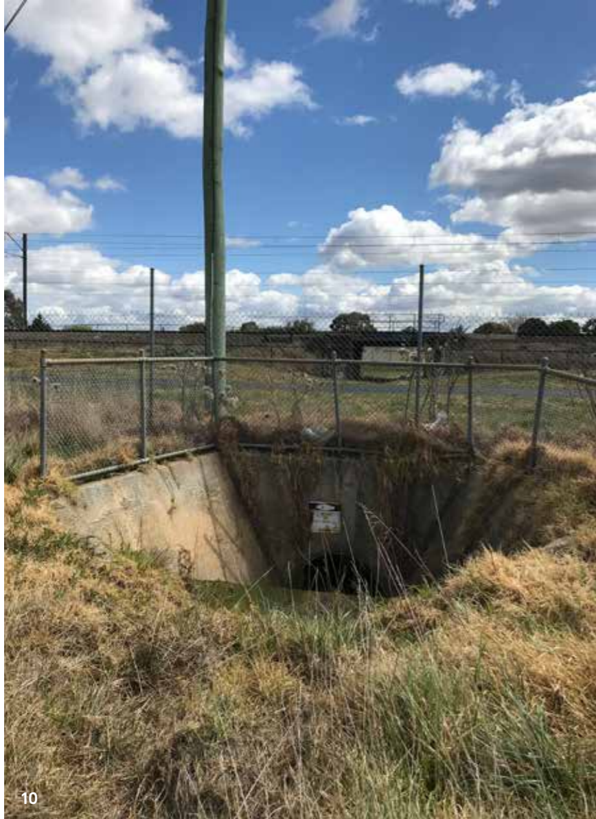
10 Existing culvert tunnel under the elevated rail on the eastern boundary of site
