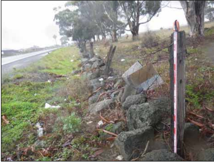
Figure 3-6: Facing south. Image showing the Dry Stone Walls that form part of H7822-0174 (Ravenhall Magazine and Storage Facility).
