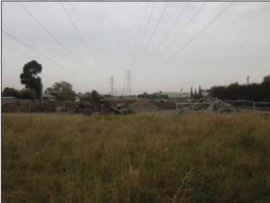
Figure 5-3: View of works currently being undertaken within the current activity area for other works.
