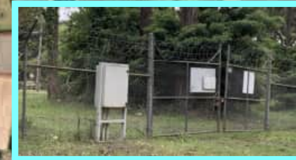
GATE 03 Cathodic Protection Pillar (Intr Rd 2 & 3)
