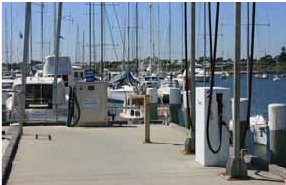
Figure 6: An example of a sewage and re-fuelling facilities (Sandringham Yacht Club)
