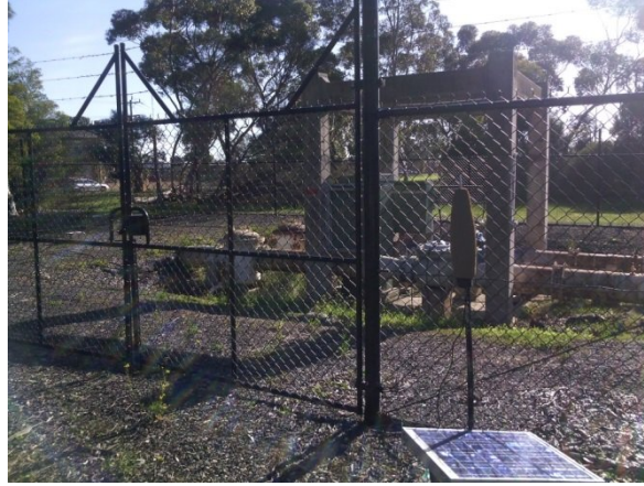
Figure 5-2: Control valves station and noise logger setup
