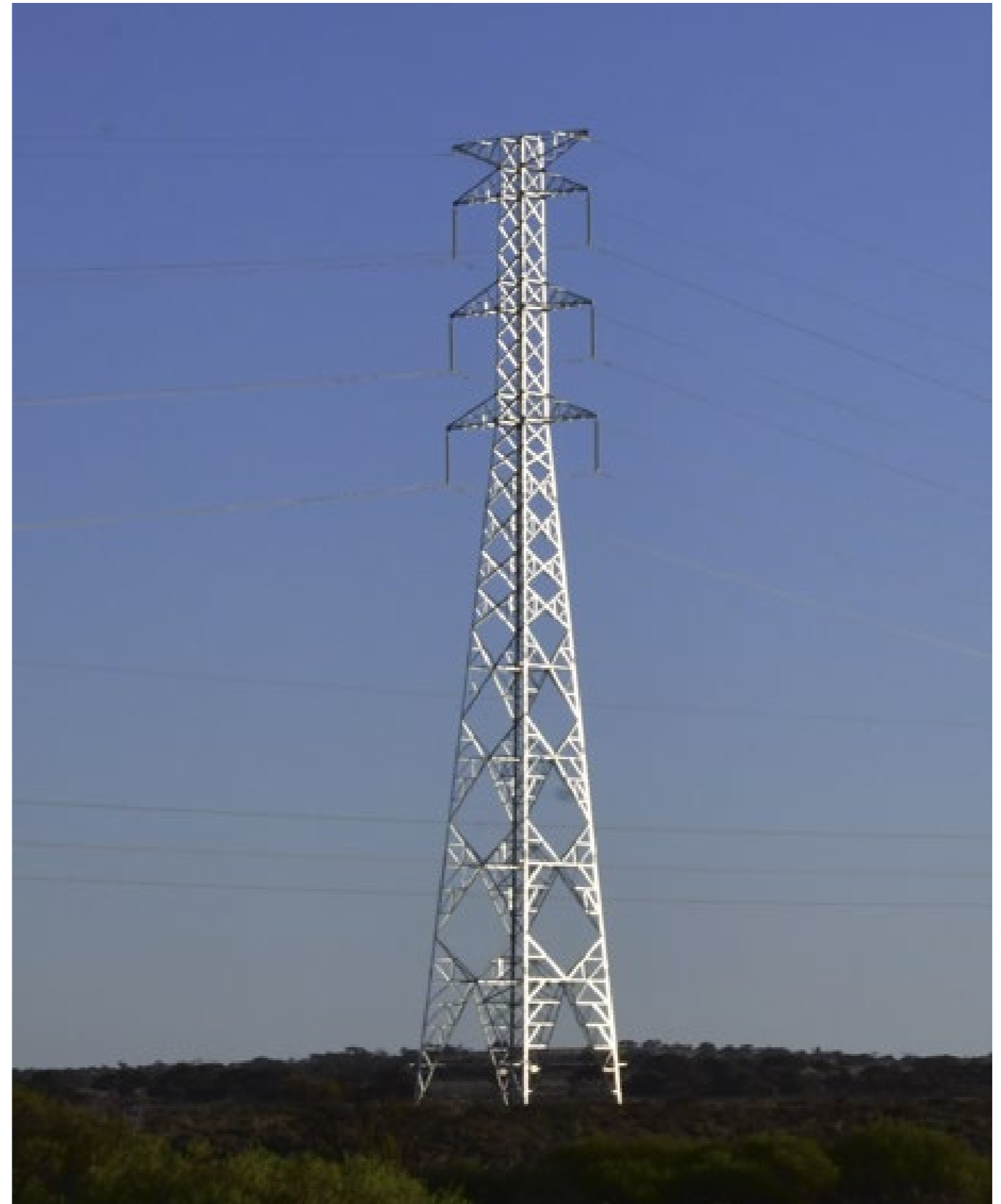
Figure 2-1 Galvanised lattice tower
