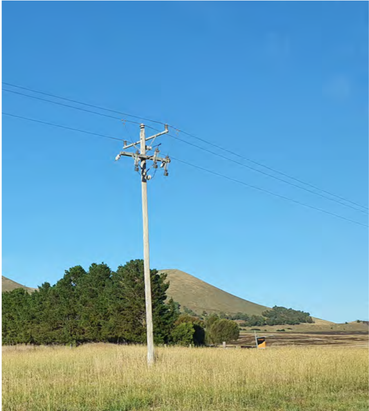
Image 3 Typical LV Power Line
