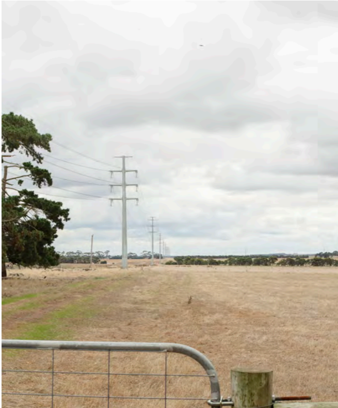
Image 2 Typical HV power line with poles
