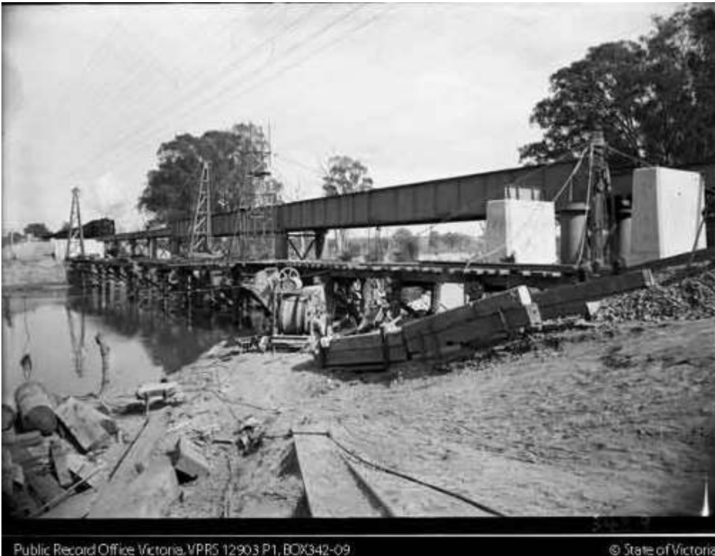
Plate 9 Construction of duplicate standard gauge bridge at Goulburn Bridge, (Public Record Office Victoria, n.d.)
