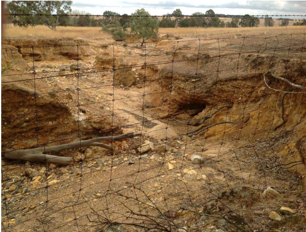
PHOTOGRAPH 7 – Erosion Washout in sedimentary units
