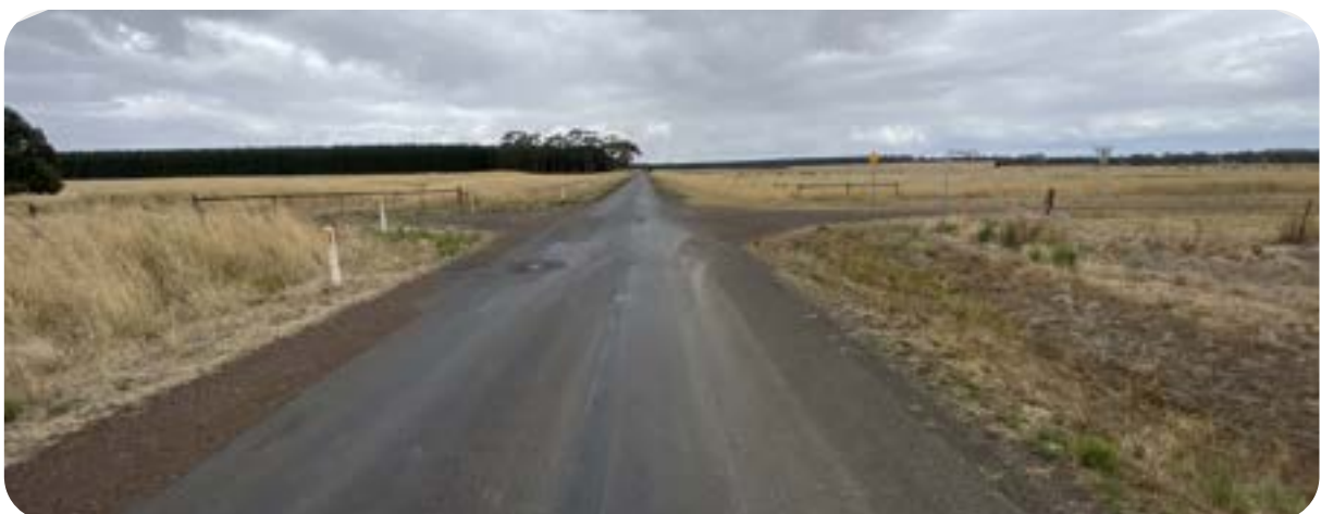
Figure 12 Mount Bute Road typical section near the subject site (Source MHWF Pty Ltd)
