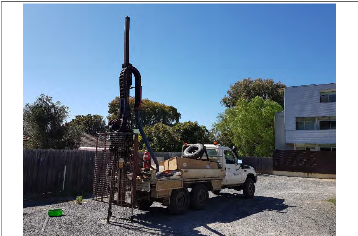
PLATE 8: Drill rig at bore SB02 in north car park – looking north-west (27 January 2017)
