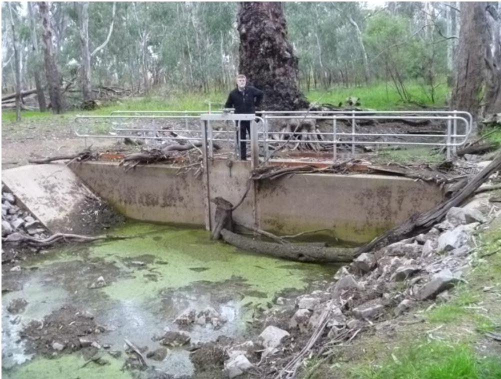
Figure 3-5 Hiskins Bend regulator looking toward the Murray River. The abutments of the structure were damaged in the 2010/2011 floods.
