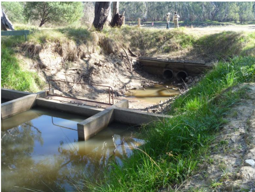
Figure 3-4 Lake Moodemere regulator looking toward the Murray River and twin culverts through the river bank
