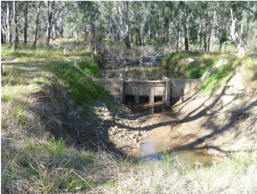
Figure 3-3 Lake Moodemere regulator viewed from the Murray River side, looking toward Lake Moodemere via the excavated channel downstream of the regulator
